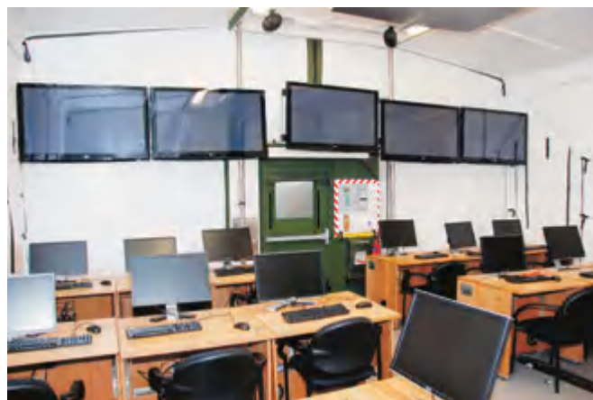
EHMECC™ Operations Centre interior.
