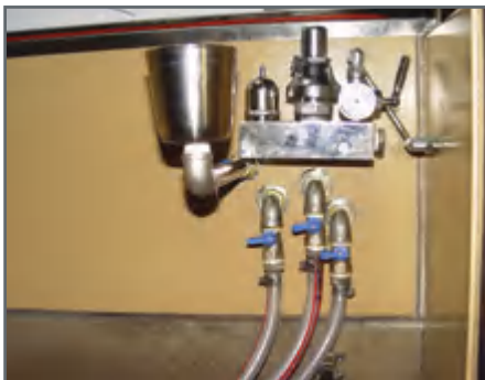
Boiling Pan Double Jacket Water Level Controlling
