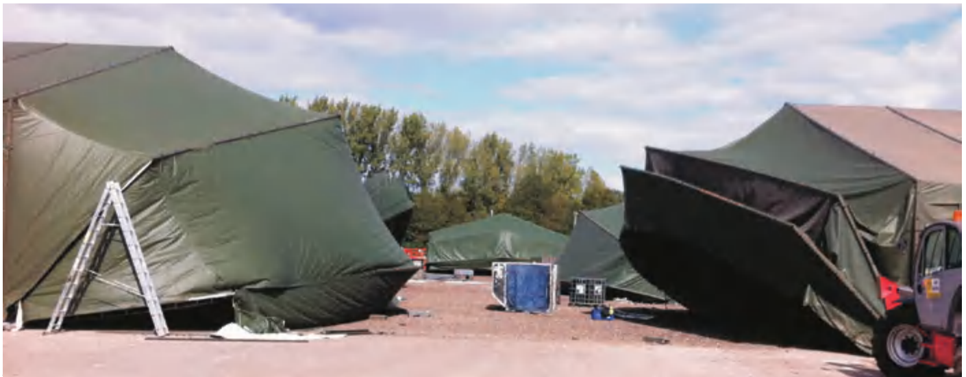
Construction site of a range of framed structures, providing support for fixed & rotary wing aircraft
